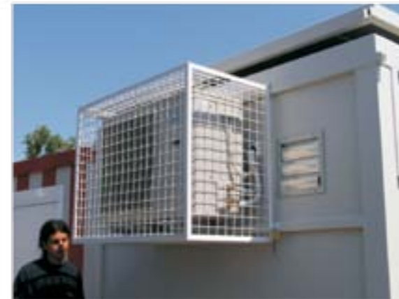
protected wire for air condition outhur unit
